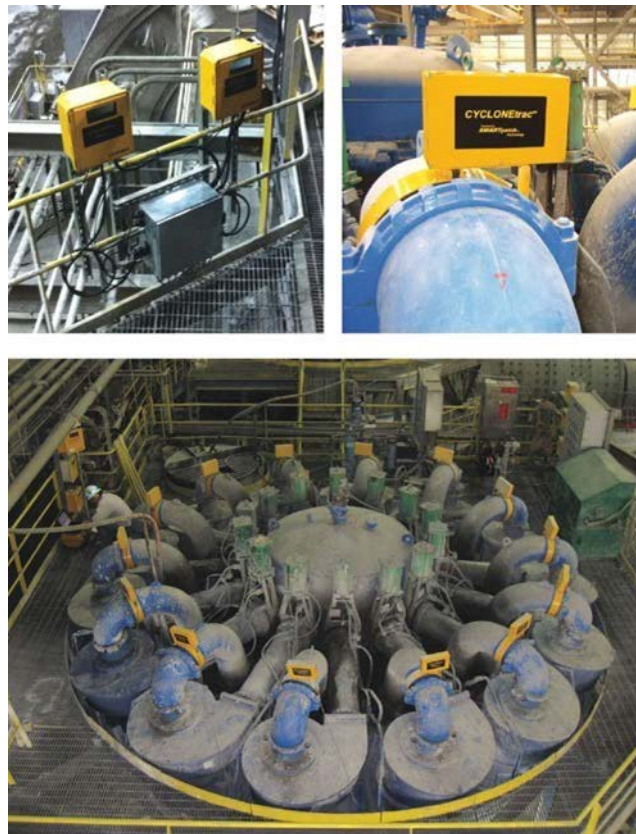
Figure 1 - Installed CYCLONetrac OSM System at Kennecott with transmitter and junction box (upper left picture), sensor head (upper right picture), and a completely instrumented hydrocyclone battery (bottom picture)
