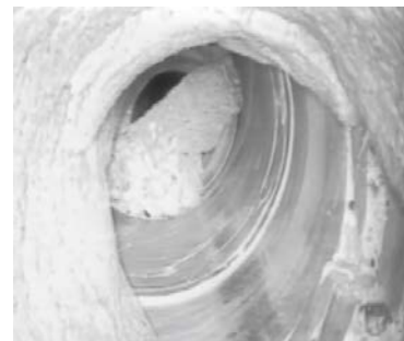
(b) surface vertical well blockage
