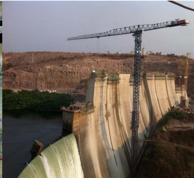
Rehabilitation and heightening by 28 m of Cambambe Arch Dam (H = 60 m), Angola
