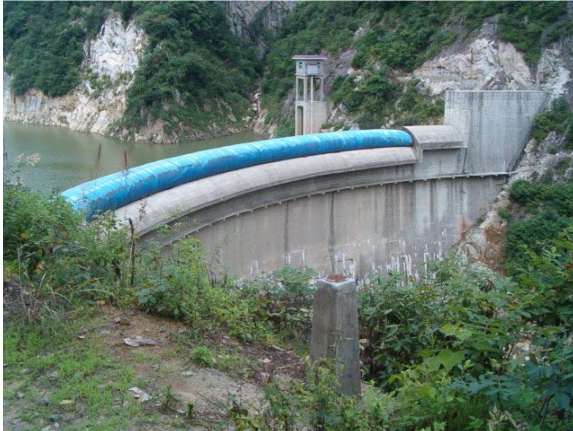
View of the Yanjia dam (Anhui Province). The dam is temporarily topped by an inflatable gate that enables a higher energy production.
