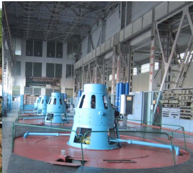
Rehabilitation of At- Bashi Hydropower Plant (4 x 10 MW), Kyrgyzstan
