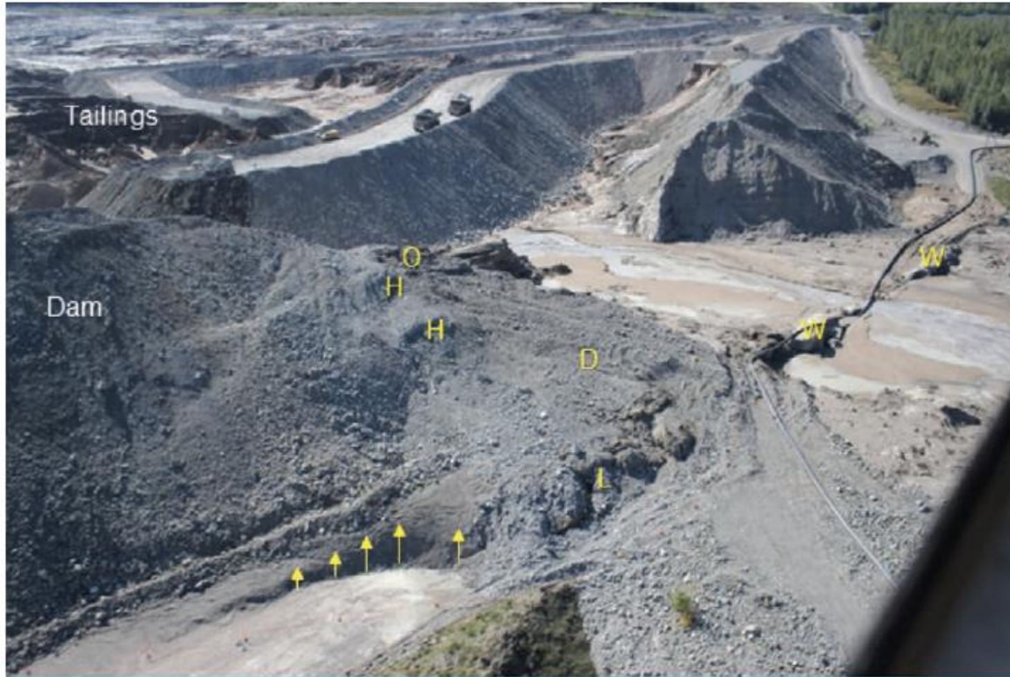
FIGURE 5.1.6: SLIDING-RELATED FEATURES AT RIGHT ABUTMENT (SEPT. 4, 2014 PHOTO)
