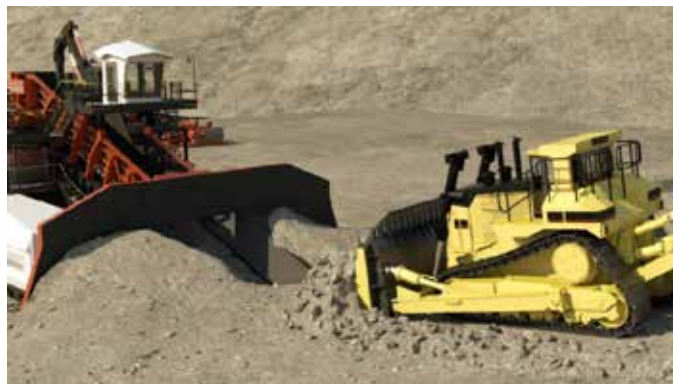
Figure 3 – Dozer pushing onto the crusher's apron feeder, with the material forming a “natural hopper”
