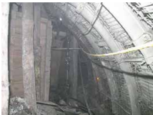
A section of the mine drift between cribs and a side wall
