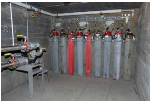
Photo 10. Methane mixture preparation chamber
