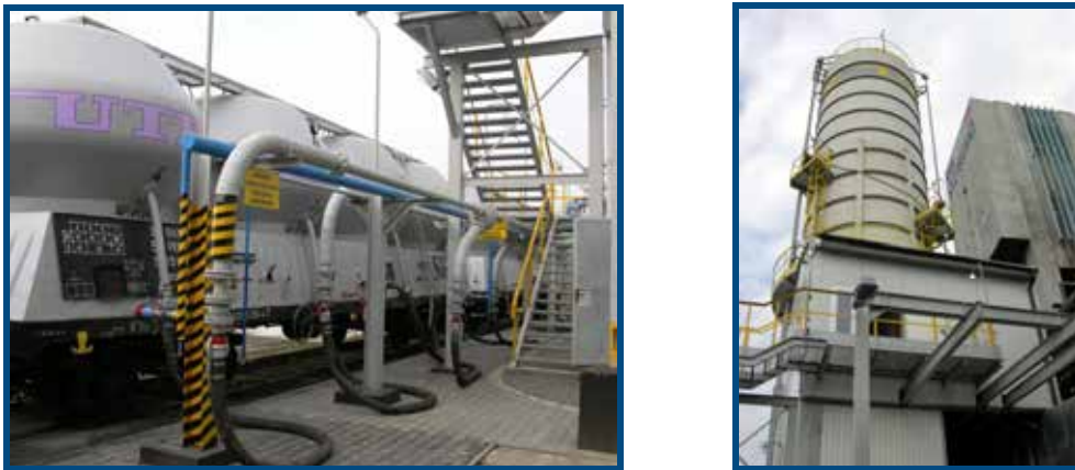
Figure 6 - Discharge of fly ash and storage tank
