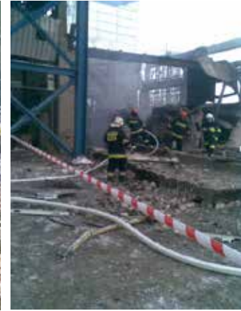
Photo 8. The Dolna Odra Power Plant after explosion
