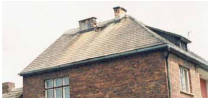
Figure 2. Characteristic damage to the buildings located in the epicentral area after the seismic event dated on 30 of September 2015 (Janina Mine)
